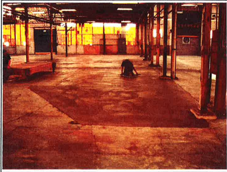
Photo No. 15: Finishing 6-inch concrete cap to match the existing slab elevation.
