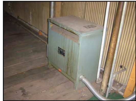
16 : Typical dry-type transformer
