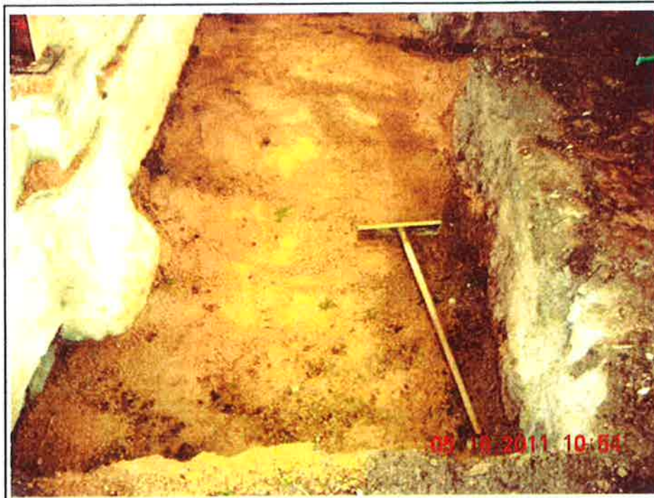
Photo No. 2: 12 inches of compacted structural aggregate in the base of the excavation.
