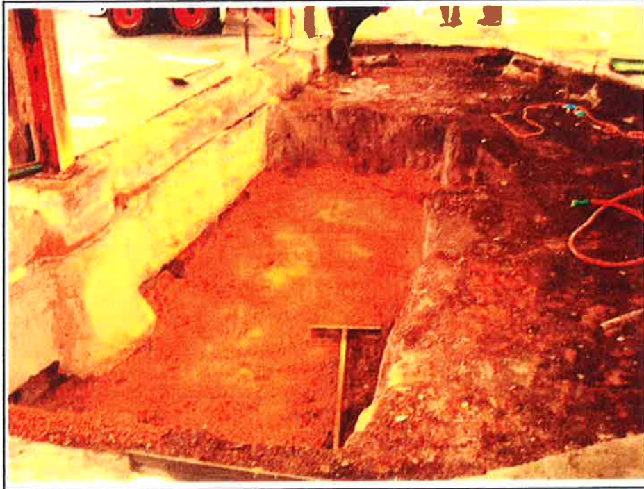
Photo No. 1: 12 inches of compacted structural aggregate in the base of the excavation.
