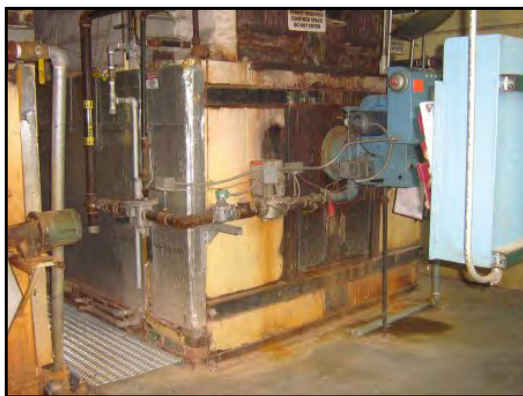
19 : Natural gas-fired boilers in manufacturing building
