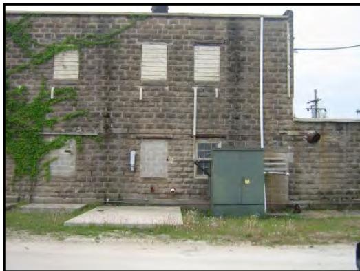
7 : North side of the foundry building and PCB-labeled transformer
