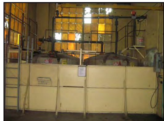
18 : Two former waste oil ASTs within enclosure
