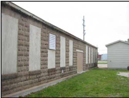
3 : Along the south side of the original portion of the manufacturing building
