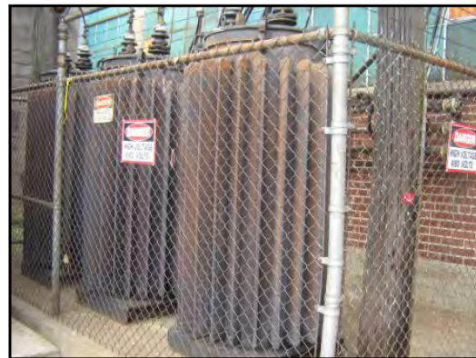
8 : Transformers on south side of the manufacturing building (labeled non-PCB)
