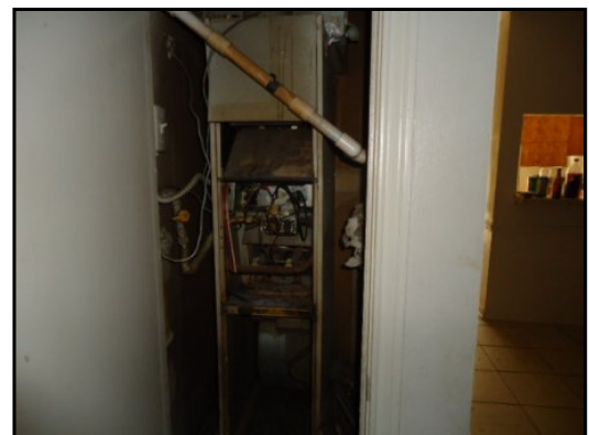
12 : Furnace contained in each unit
